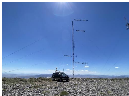
150 ft tower with 4 UHF antennas / transmitters
